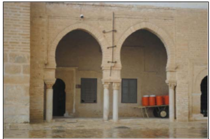
Figure 4. Two retrofitted arches in the Kairouan Great Mosque. The two retrofitted arches show different structures with the lower left structure and distorted right arch. Pillar tops are not at the same level, and the two structures are clamped with three iron hooks. The color version of this figure is available only in the electronic edition.
