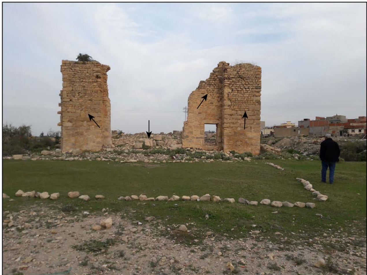
Figure 6. Damaged Roman city of Cululis (now Ain JIoula, see location in Figs. 1 and 2a,b). Arrows on frontal wall show the different building stones with evidence of reconstructions and
